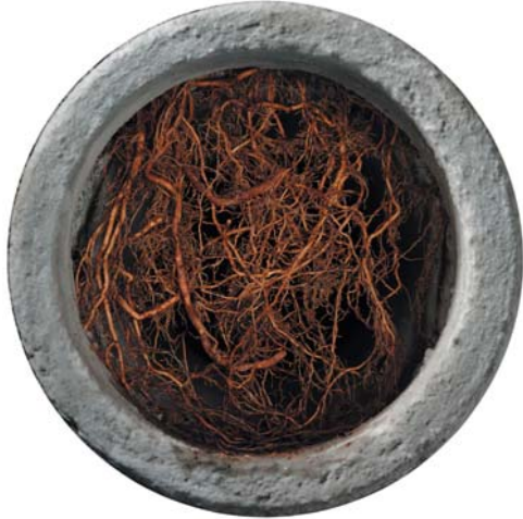
Rootlets in Sewer
