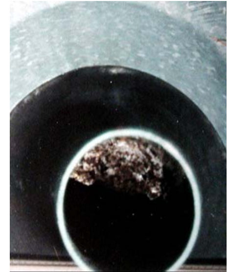
Roof Vent with Debris
