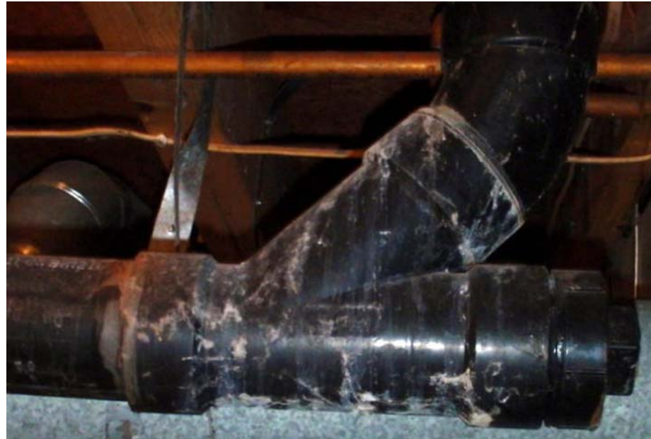
Visible Leakage from Sewer Pipes
