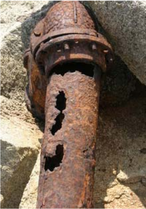
Corroded Sewer Pipe
