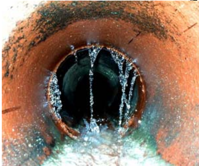
Leaking terra cotta sewer pipe
