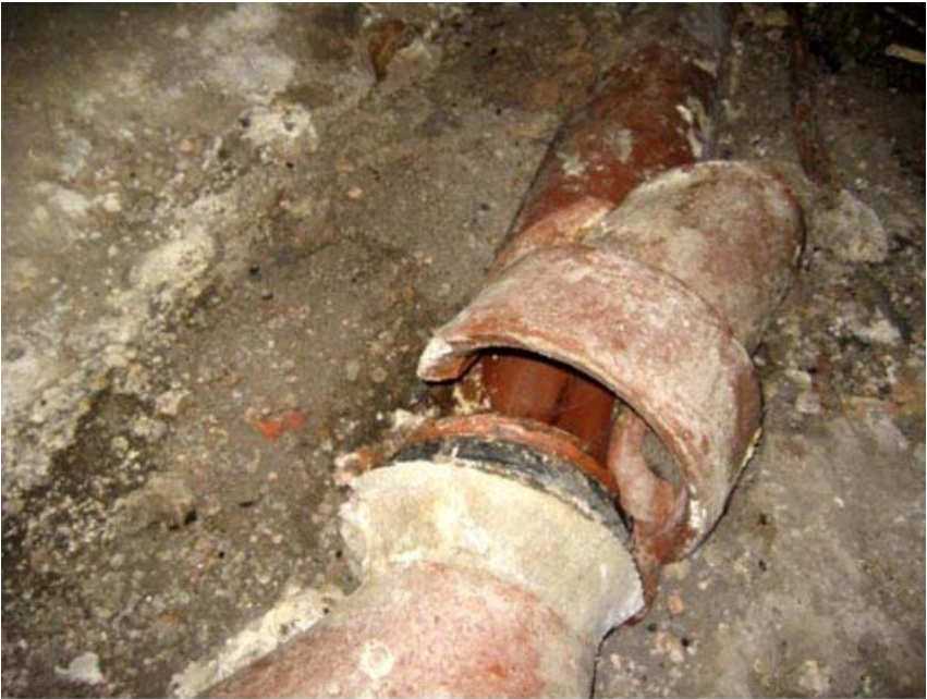
Separated Sewer Pipe
