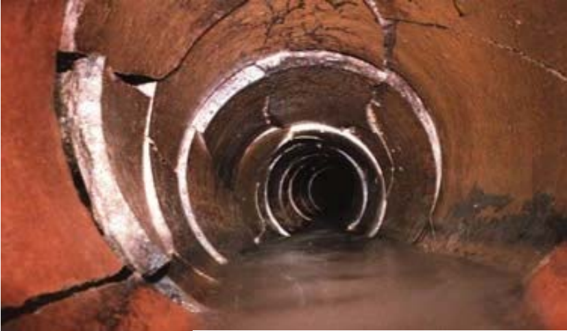
Cracked Sewer Pipes
