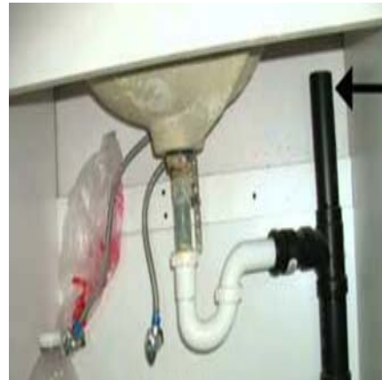
Vent under Sink
