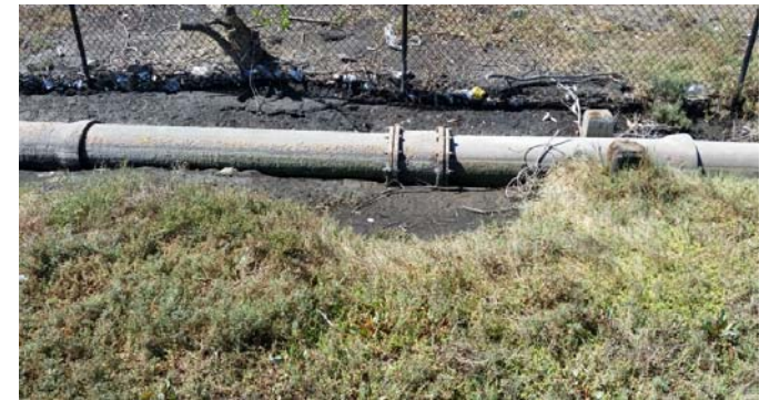
Cast iron pipe
