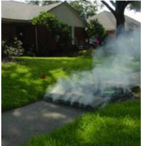
Smoke locates sewer leaks
