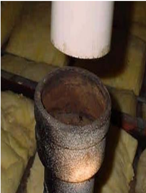
Misaligned Attic Vents
