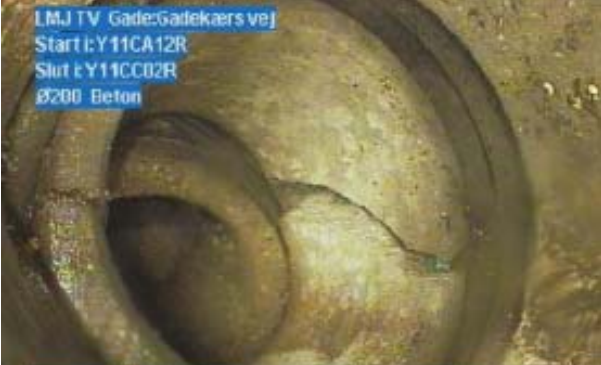
Cracked Sewer Pipe (Riis)
